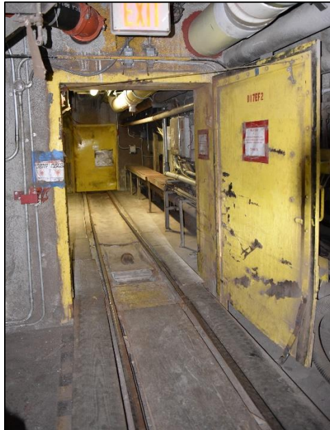
Figure 1: Image of open oil-tight door (foreground) and closed ventilation door on either side of the damaged fire suppression system low point drain valve. [Encl (169)]
