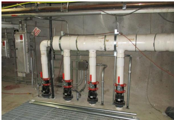
Original AFFF Retention Line Piping in Immediate Area of an AFFF Sump
